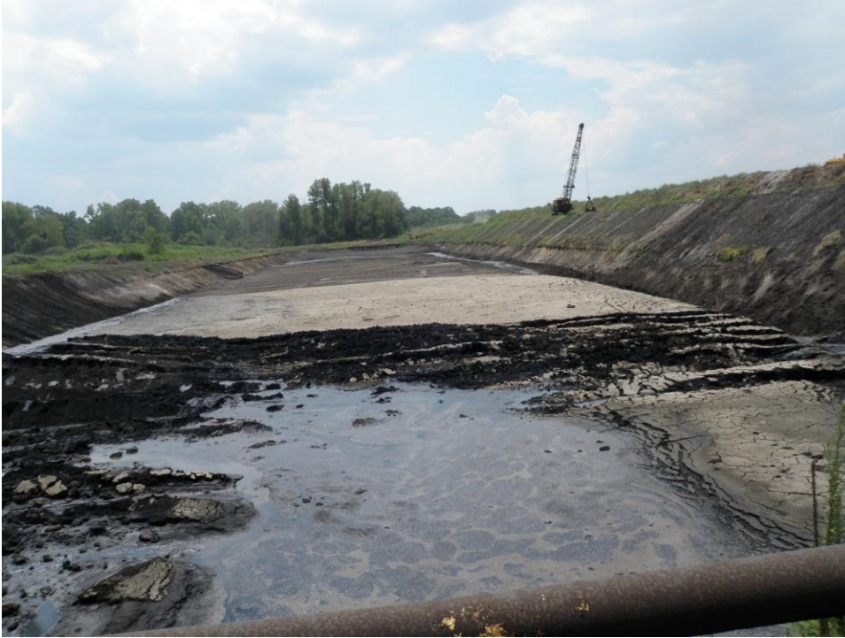
West Ash Pond – permittee is in the process of cleaning out solids
