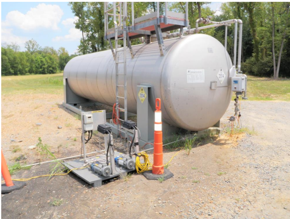
Hydrogen Peroxide and Iron catalyst feed system at clarifier.
