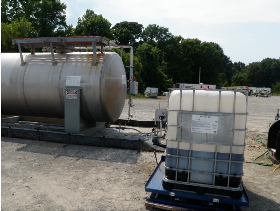
Hydrogen Peroxide and Iron catalyst feed into P2 sewer
