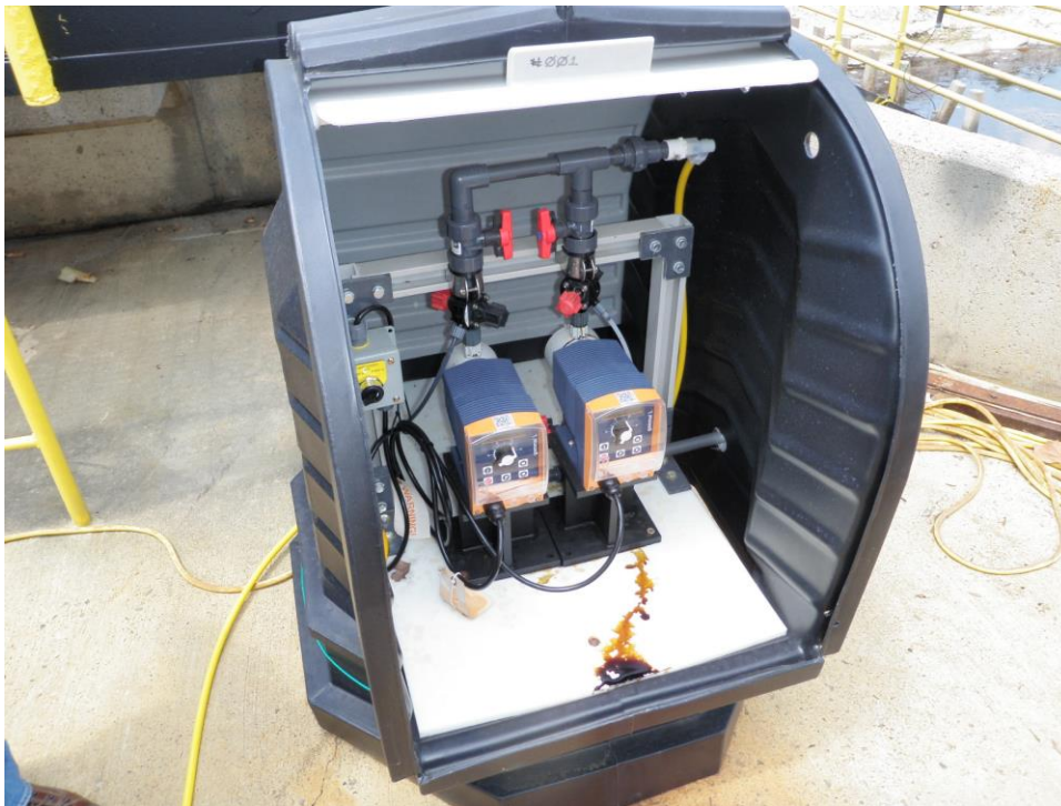
Pumps for feeding Hydrogen Peroxide and Iron catalyst at clarifier.
