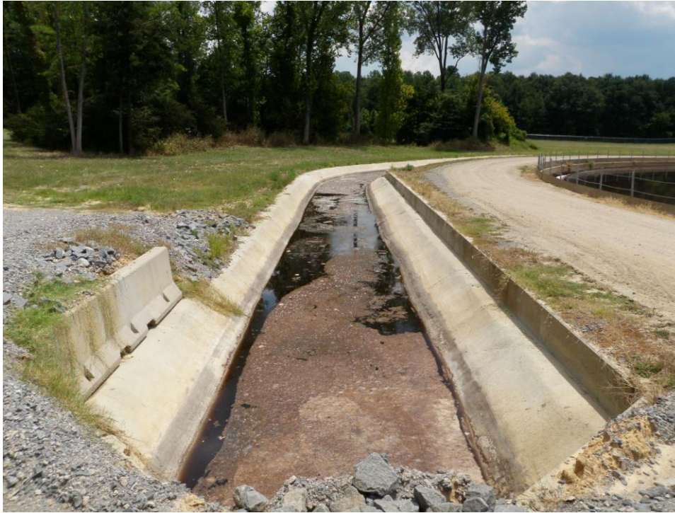
Clarifier Bypass. This is used only in emergency situations.
